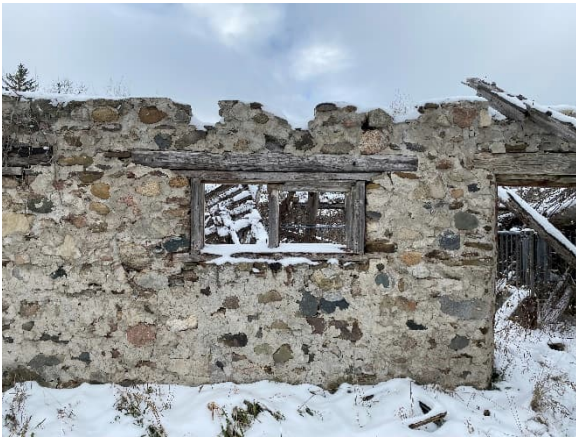
Plate 23: Parged fieldstone wall and window
